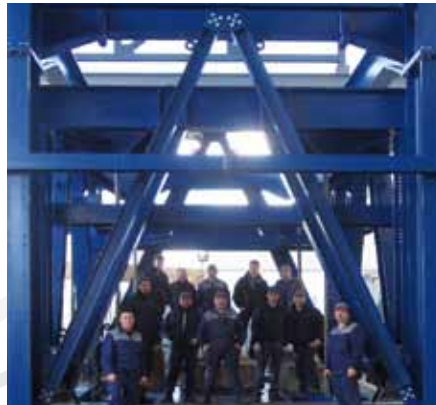
MAURER FOLDED PENDULUM DAMPER INSTALLATION TEAM, SOCAR TOWER, BAKU
